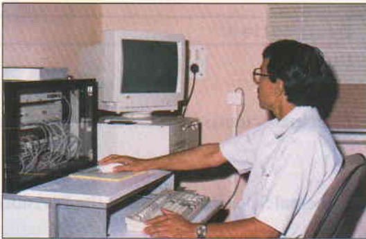
Local Area Network (LAN) facility at the Institute
